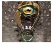
Part of the detection element has 'hung up' on the deflector plate which in turn stops the water dispersing correctly.
