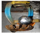
The fusible element has dropped and hung on the deflector plate, which in turn stops the water dispersing correctly.
